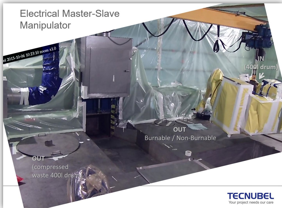
Figure B.28. EMS, wrapped in yellow foil, on mobile bridge above the working platform in a double tent confinement, equipped with a 100 tonne press (photo ENGIE Tihange Nuclear Power Plant )
