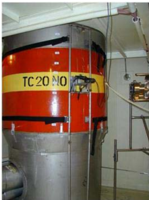
Figure 51: Activity profile measurement of primary clean-up filter at Czech NPP Temelin
