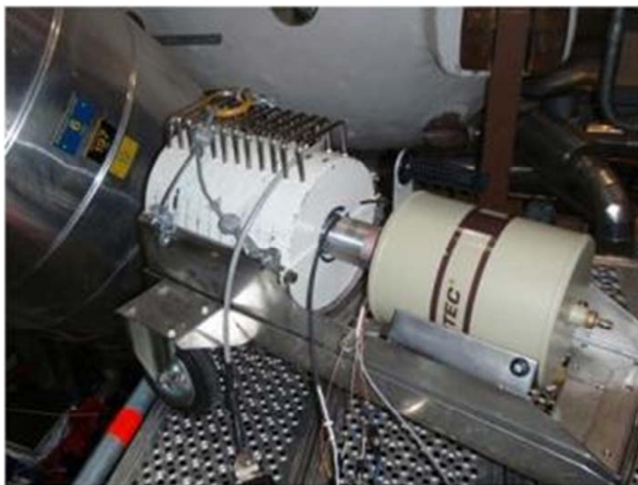
Figure 56: Portable HPGe detector with collimated shielding for a BWR MADAC based measurement campaign, here measuring on a BWR-75 steam pipe (Forsmark 3)
