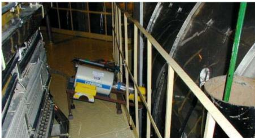
Figure 50: Steam generator measurement at Hungarian NPP Paks
