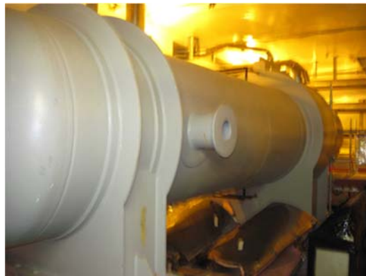
P8: RHRS - Heat exchanger
