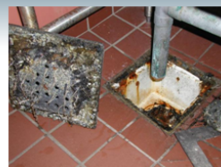
Dirty floor drains create food safety risk.
